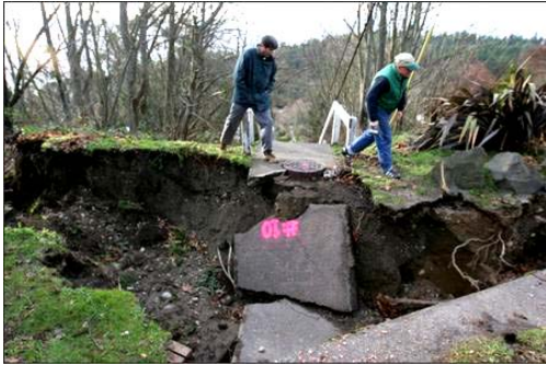
Sinkhole causes flooding in West Seattle Jackson's backyard a few hundred feet away. (December 15, 2006)
